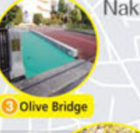
3 Olive Bridge You can walk over it, but it is under construction until July 2018.
